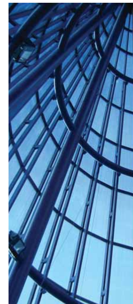
Khalifa Stadium in Doha, Qatar using Lexan Thermoclear SunXP 25mm sheet in blue
